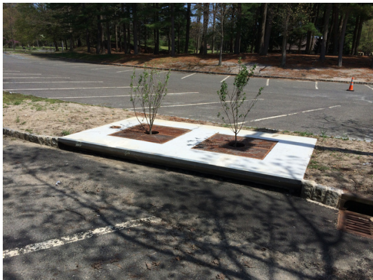
An example of GSI in Ocean County Park, New Jersey using a Filterra Tree box biofiltration system that has been optimized for high volume/flow treatment and high pollutant removal. Photo credit Princeton Hydro LLC
